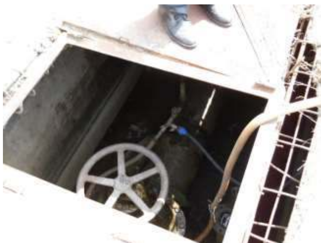
Camin vane iesire SP repompare – spre distributie
