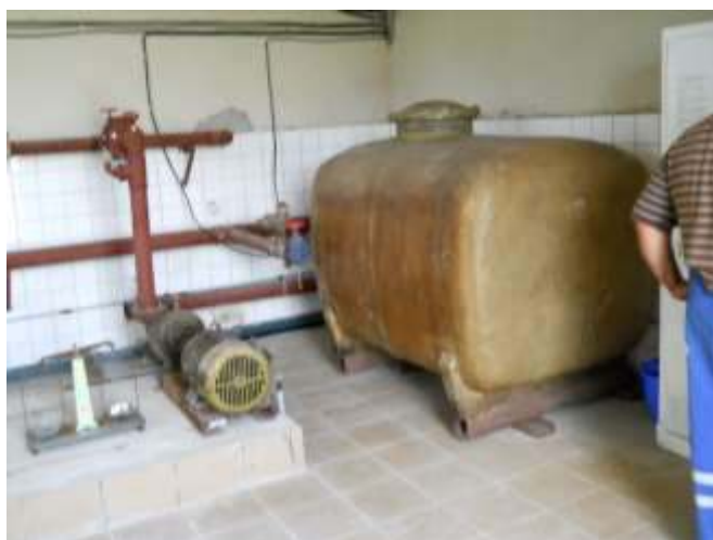
SP re-pompare Corabia - “Laborator analize”
