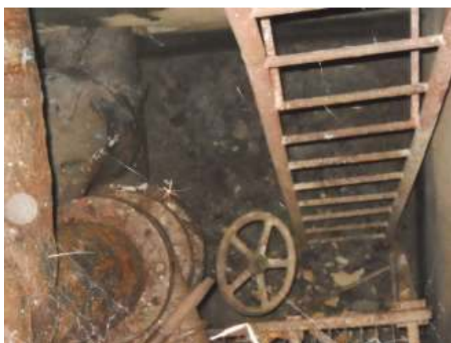
SP Re-pompare Corabia – aaces sala pompelor
